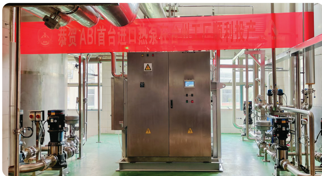
Onsite photo of the Heat Pump operation [Banner headline: Congratulations on the first imported heat pump successfully put into operation in Taizhou factory.]
