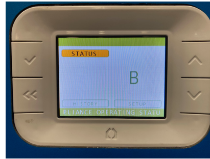
BDB—Boiler Display Board
