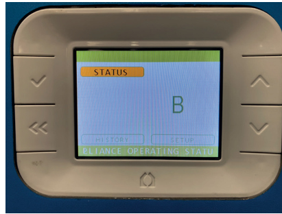
BDB—Boiler Display Board
