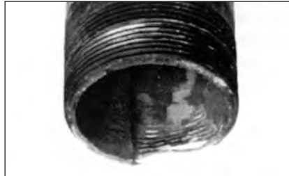
Figure CG-9. CO 2 gas combines with condensate allowed to cool below steam temperature to form carbonic acid, which corrodes pipes and heat transfer units. Note groove eaten away in the pipe illustrated.
